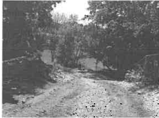
Photo 2. Access road cut into bank. Looking down slope from upstream of gate chamber.
