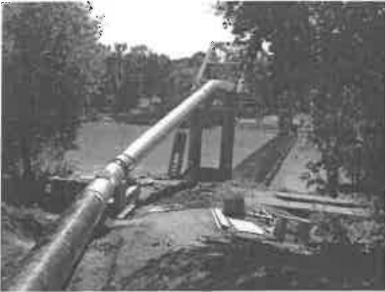
Photo 1. Construction activities on pipeline and bridge. Looking down slope from lift station.
